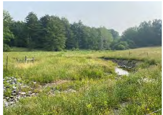
The armored spillway and eroded bank, starting to recover in the fenced riparian area. Image: USFS
