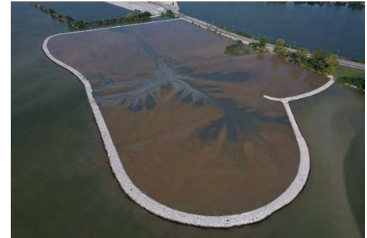
Sediment placement within a constructed wetland is the first step in creating new in-water wetland habitat in Sandusky Bay. Image: USACE
