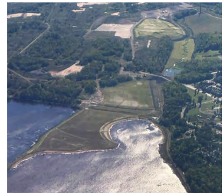
Aerial view of Spirit Lake project features, including new shallow sheltered bay, delta upland cap and the upland confined disposal facility. Image: EPA
