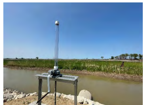
Pictured is the installed fish passage structure that provides access for fish from Lake Erie to the John Gradel Marsh for spawning and feeding. Image: Courtney Lopez, USFWS
